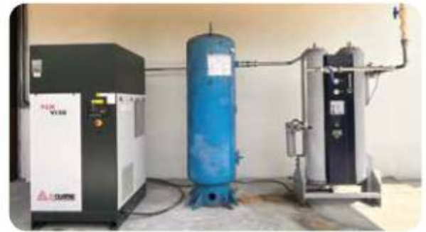
Oil Free Compressed Air System
